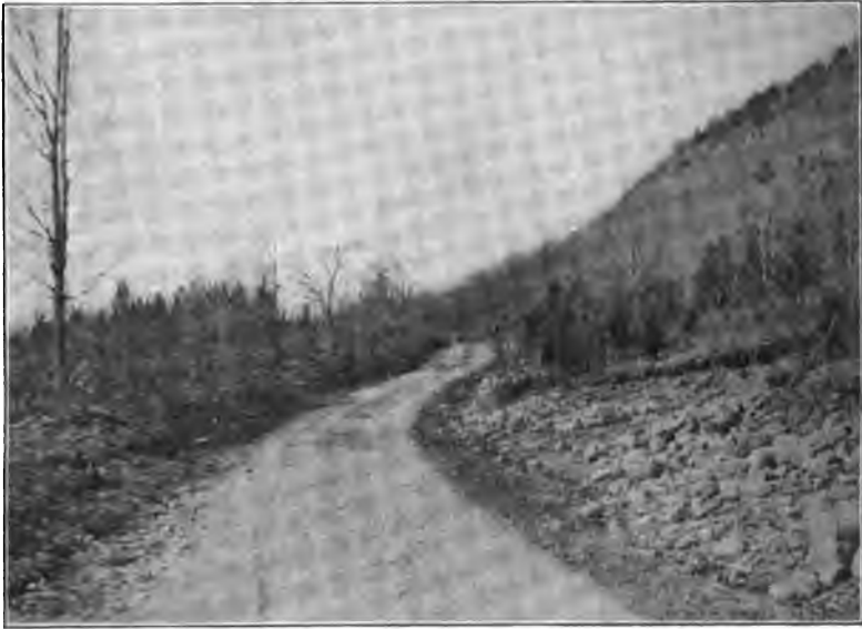
Macopin road, Passaic Co., from Butler, N. J., before improvement.
